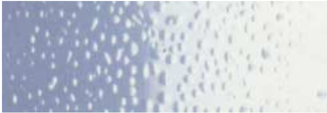
FIGURE 28-8 Paint blistering is normally caused by excessively fast solvent evaporation.
