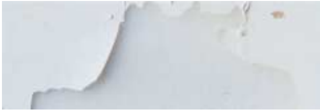
FIGURE 28-12 Peeling is a catastrophic paint failure of older finishes.
