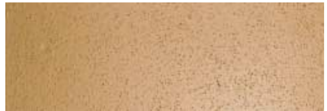
C Sand in the finish can occur if areas were sandblasted during rust repair and someone did not blow out all of the repair areas to remove all sand before painting.
